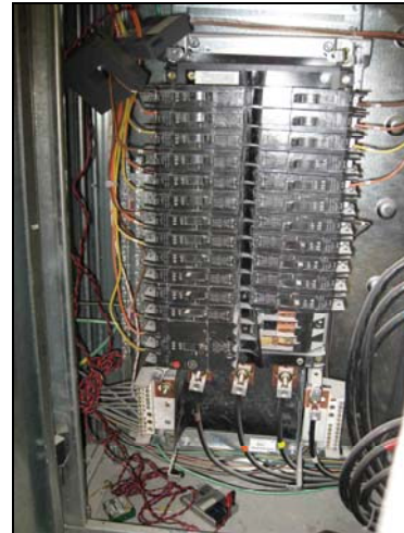
FIGURE 2-4 – LIGHTING PANEL HA WITH MONITORING EQUIPMENT
